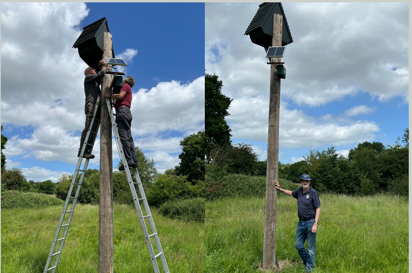
Colin and Duncan fit the wiring then Ted holds up the pole!!
